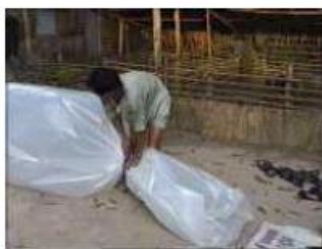
Photo 30. Tying the tube but leaving enough plastic to insert the outlet pipe
