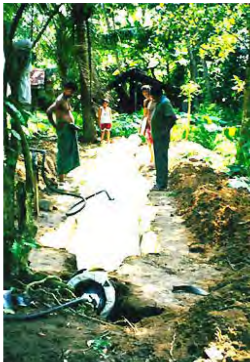
Fig 1. The biogas plant. Gampaha, Sri Lanka
