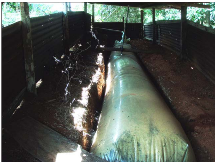
An in-ground bag digester in operation. Photo by Ian Woofenden.
