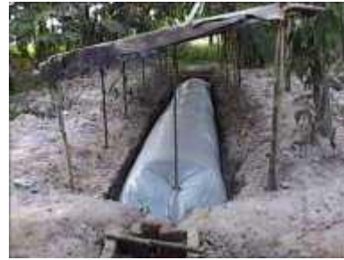
Photo 69. Roofing can protect the biodigester
