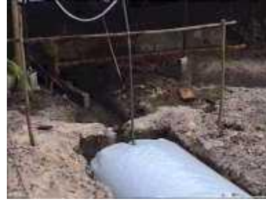
Photo 65. The channel is connected to the biodigester
