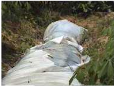
Photo 81. The outer plastic layer damaged (after 3 years..!). The inner one is still gas-tight.
