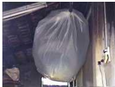
Photo 59. The reservoir bag full of biogas
