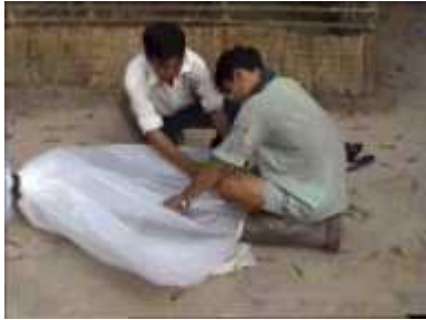
Photo 31. Placing the outlet pipe (following the same procedure as for the inlet pipe)
