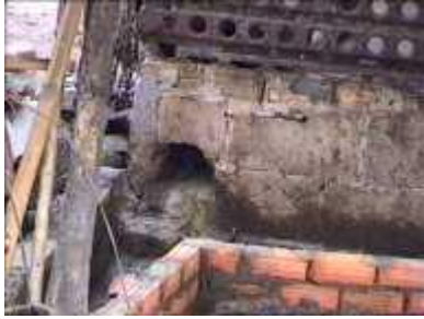
Photo 64. A channel is made with bricks to lead the waste from the pig pen to the inlet of the biodigester
