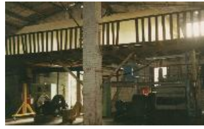
Photo 98. A large reservoir bag provides biogas for a diesel generator in the integrated farm of Pozo Verde, Colombia
