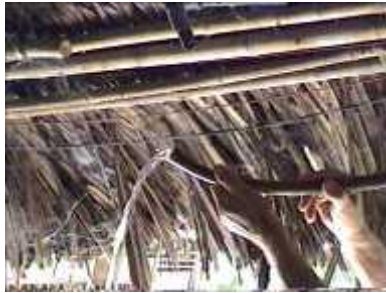
Photo 78. Accumulation of water. Open the joins and take out the water as it can be accumulated (# 6-1)
