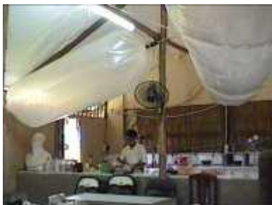
Photo 95. Reservoir bags storing biogas in the the laboratory of UTA
