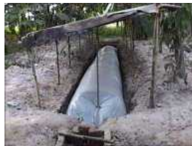
Photo 69. Roofing can protect the biodigester
