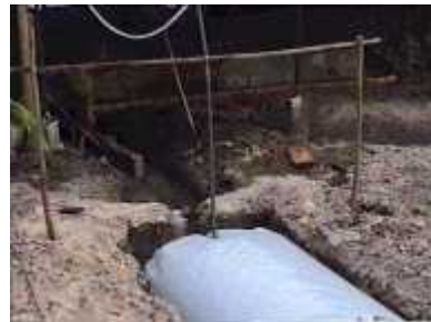
Photo 65. The channel is connected to the biodigester
