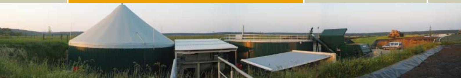
Photo 13: General view of a two-step, 500 kW el only energy crop digestion plant with digester 1 and dosing unit (center), digester 2 with integrated gas holder (left), silage clamps (background) and storage lagoon for the digestate (foreground right).
