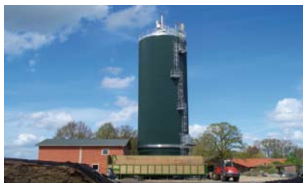
Photo 15: The dry-digestion installation with the feeding bin from where the digester is fed automatically
