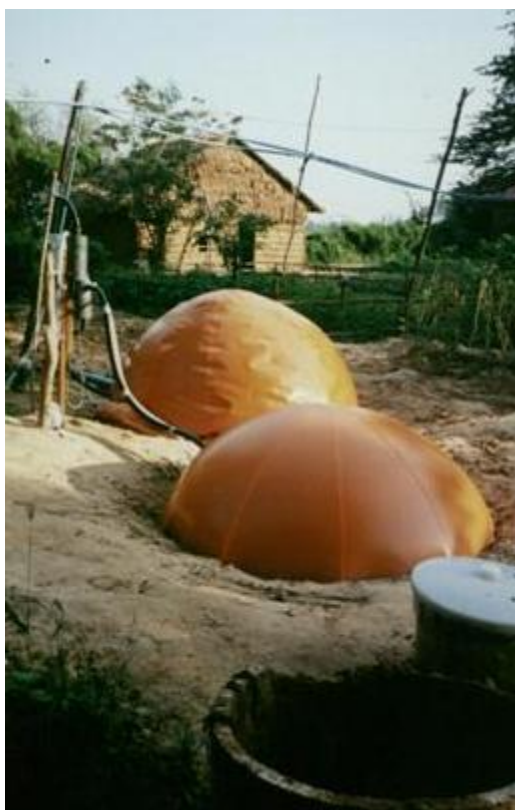
Figure 3: The “super-gas” mixing biodigester installed in UTA, Cambodia
