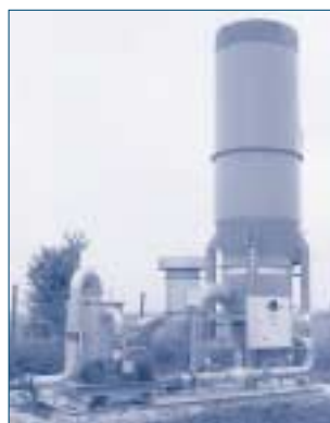
Figure 2.6 | Example of a forced air enclosed flare
