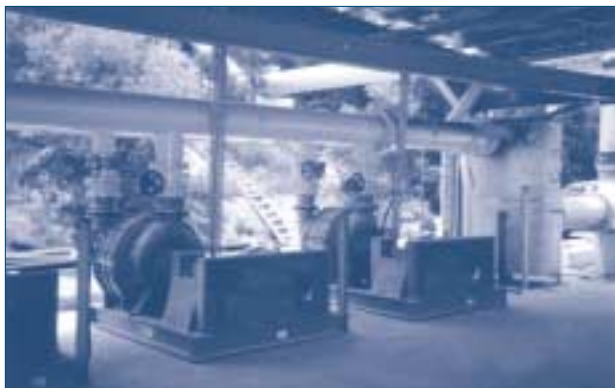
Figure 4.2 Duty/standby gas boosters after a moisture removal pot
