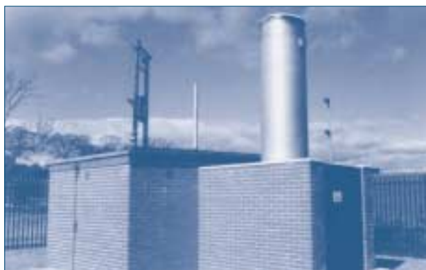
Figure A5.1 High-temperature, low-emissions enclosed flare within a brick enclosure to reduce noise impact
